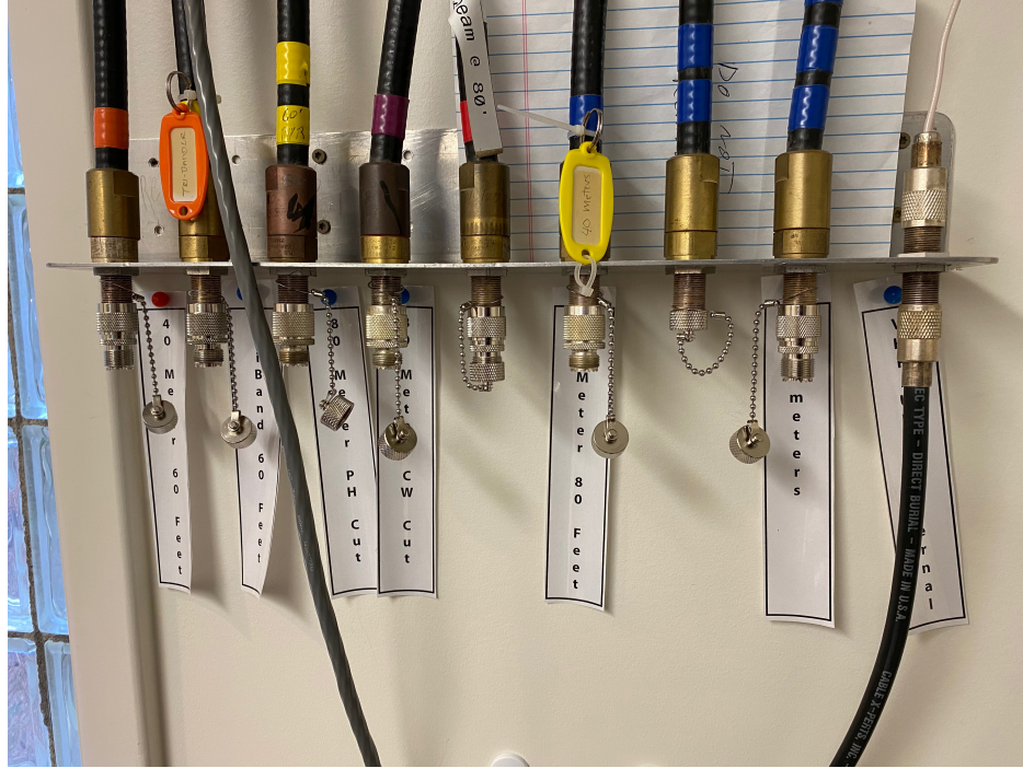
Figure 11.7.: Antenna connections in clubhouse interior
